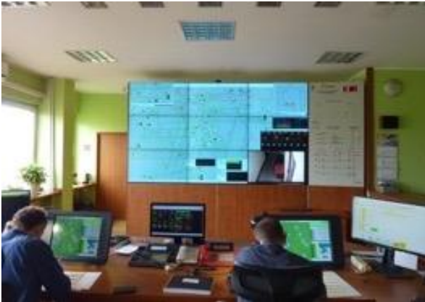
Ventilation control room
