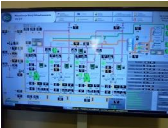
Methane drainage monitoring
