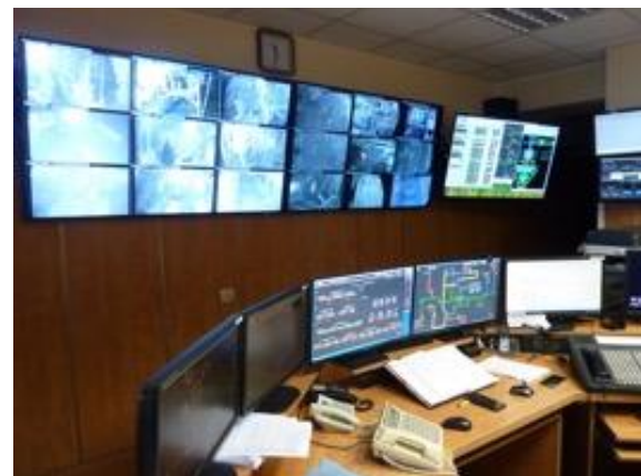
Engineering control room
