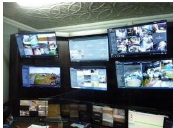
Security control room
